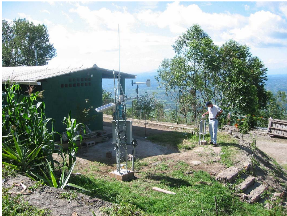
Fig.1 Installed rainfall station (San Vicente)
